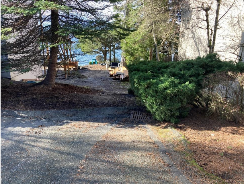
Photo 1: Looking West from the end of Bonney Street. Note the final stormwater catch basin before system outfalls into Lake Washington.
